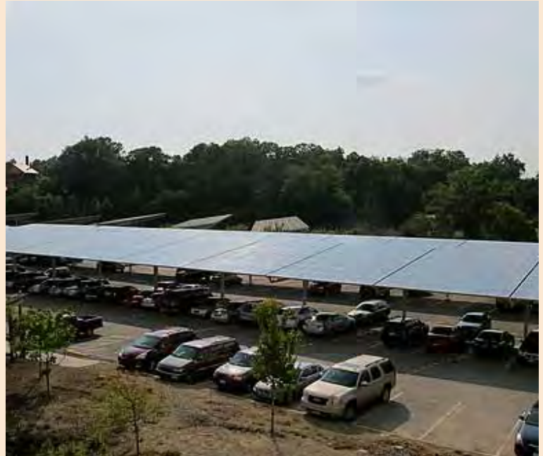
Solar canopies at the Cincinnati Zoo generate 1.6 MW of energy
